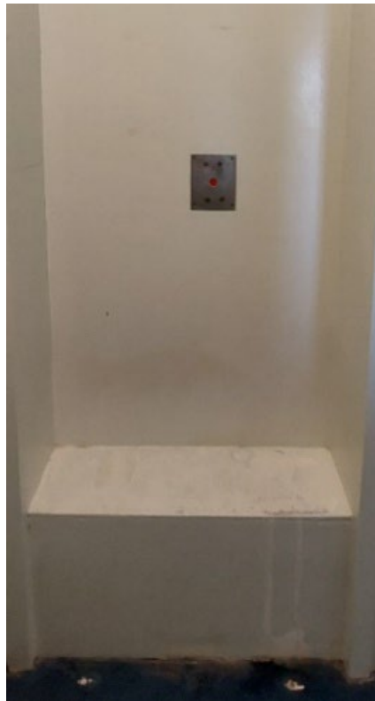
Image 4: Duress alarm in shower
