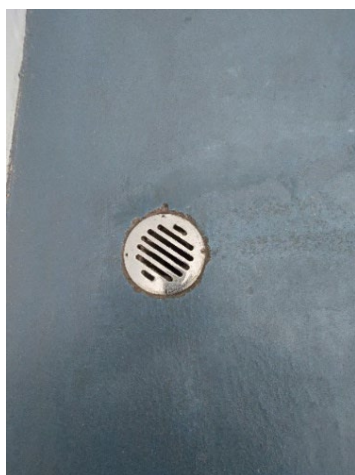
Image 12 Cell Holding cell drain assembly
